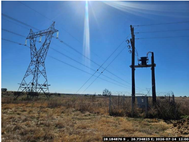
View of the 33 kV powerline connection point at the compressor station
