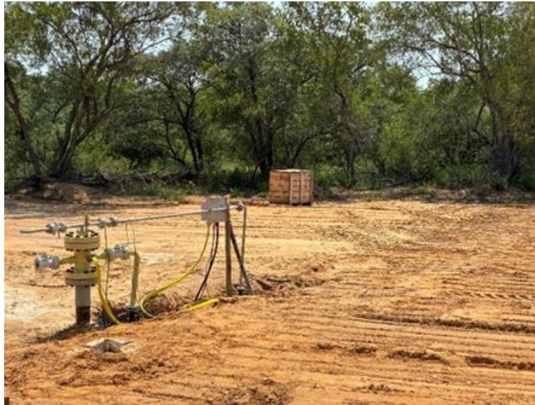
Figure 8: View of typical production well above ground infrastructure.
