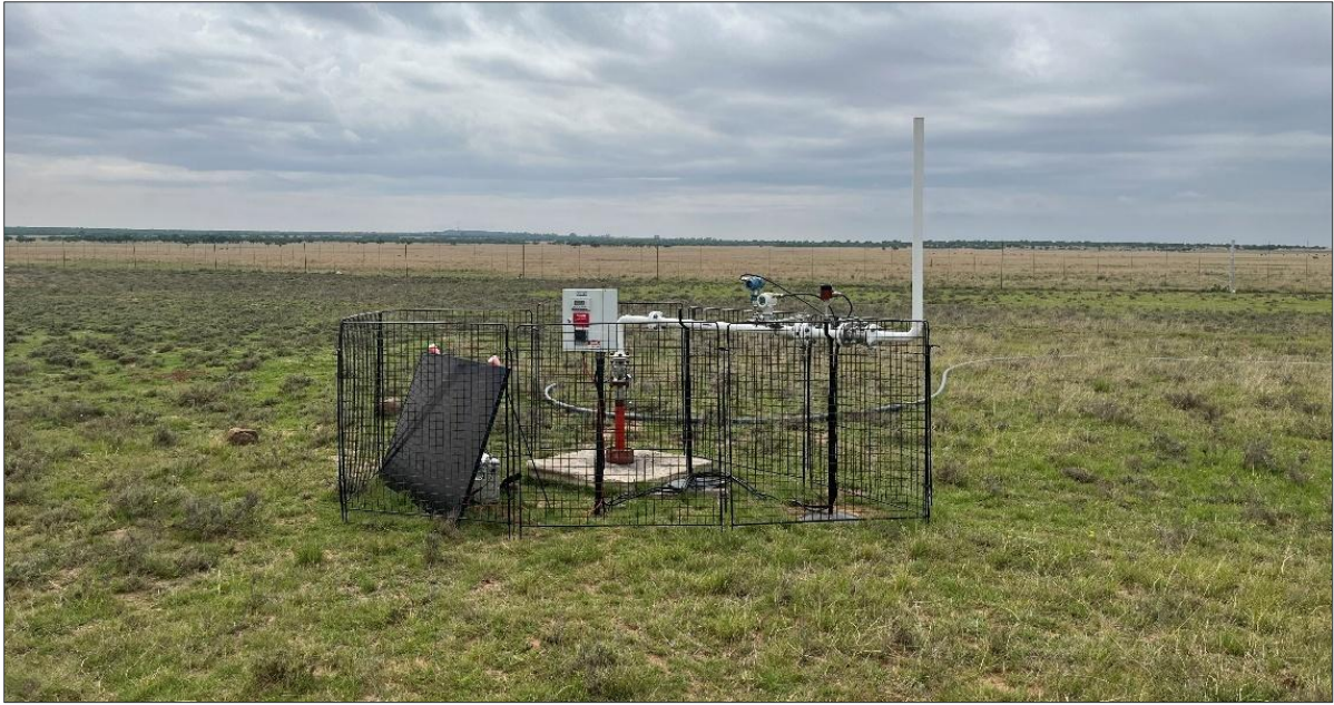
Figure 8: Typical wellhead surface infrastructure (to be connected to underground pipeline if converted to production well).
