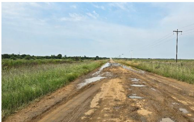
Figure 23: Some of the infrastructure within the ER include surfaced and gravel roads. The conditions of the roads vary from good, maintained roads to roads which have been severely deteriorated roads in poor condition.
