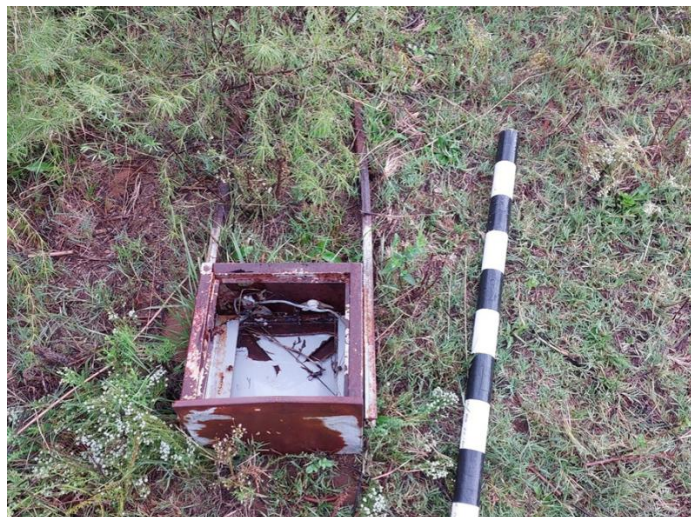
Figure 45: Telephone junction box found at MO002
