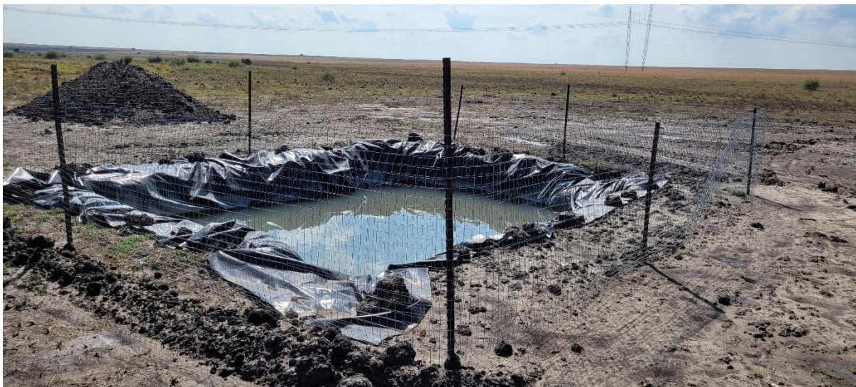
Figure 105: Typical traditional sump pit used for one of the approved D3 Energy drilling sites in the region.
