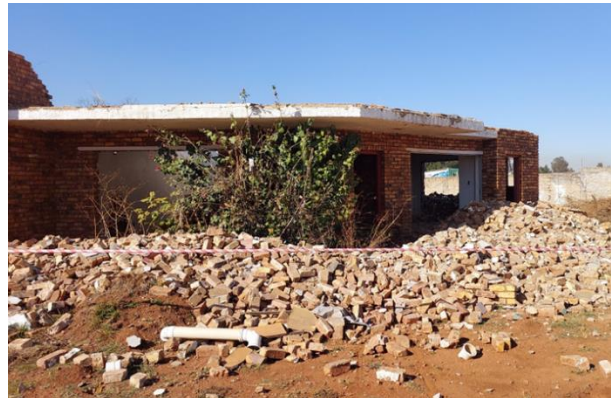
Figure 10: Dilapidated buildings to be demolished.
