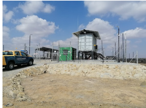
W – Tetra4 Compressor Station
