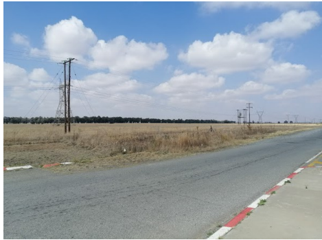
SW – The 132 kV LILO is to be connected to the 132 kV powerline spanning across on the image above.
