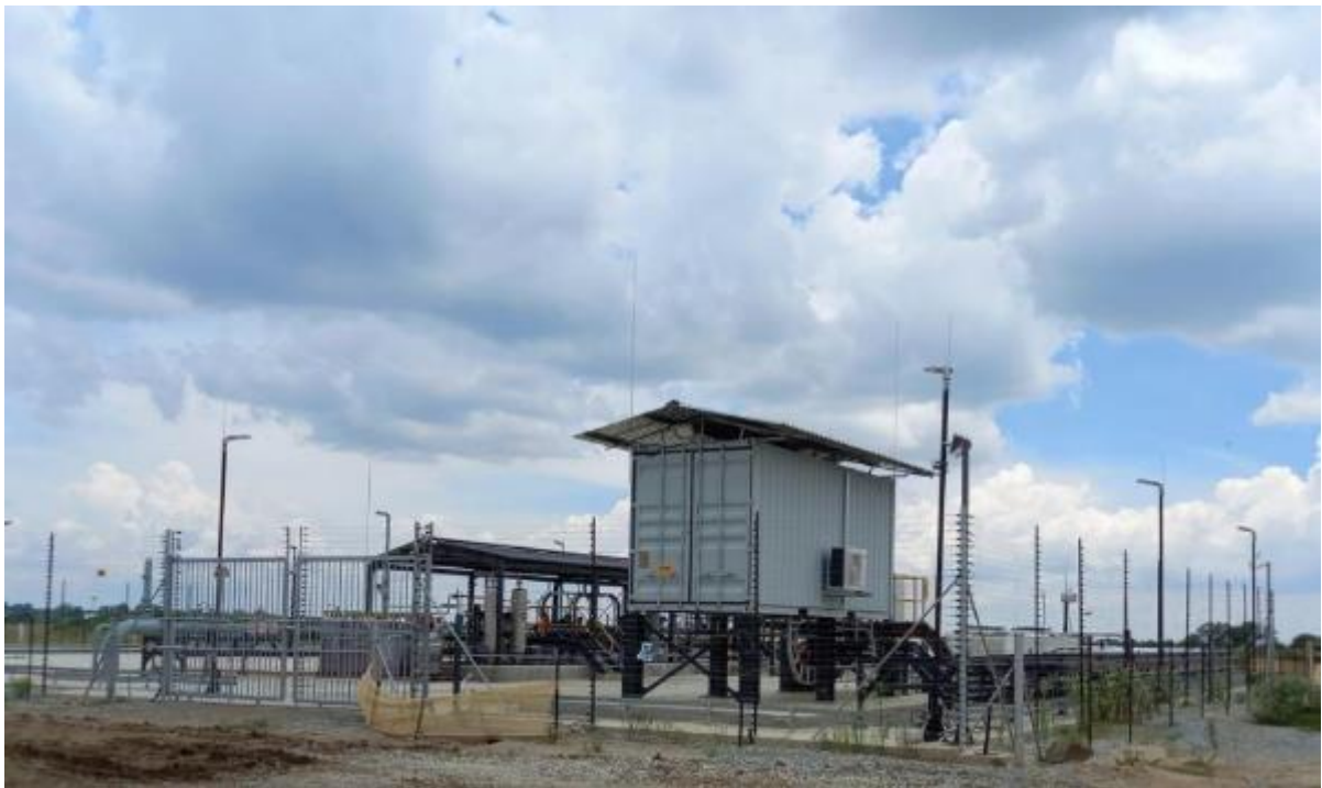
Figure 11: Example of Compressor Station just recently constructed as part of Cluster 1.
