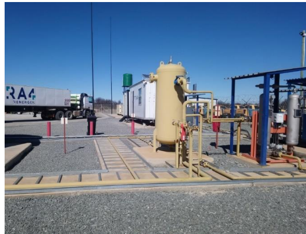
Figure 18: HDR1 Production well and associated facility.
