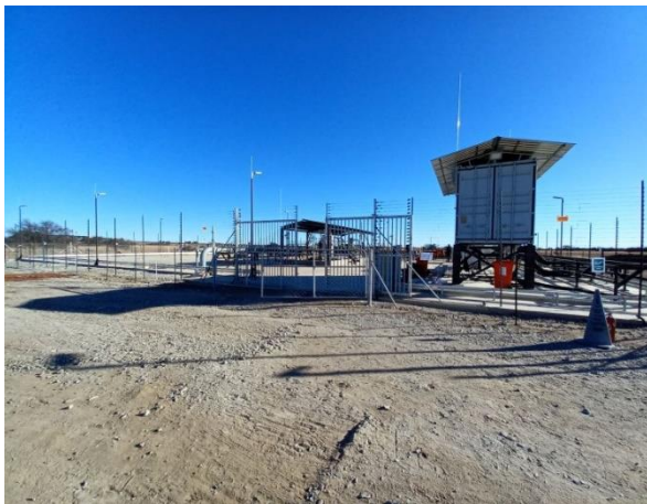
Figure 11: Centralised Compressor station.
